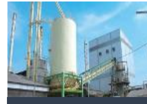
Biomass Co-Generation System, Fuji-Foods Coporation, Thailand
