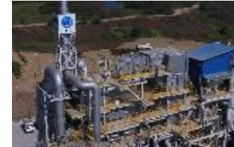
Waste to Energy Plant, JFE engineering, Myanmar
