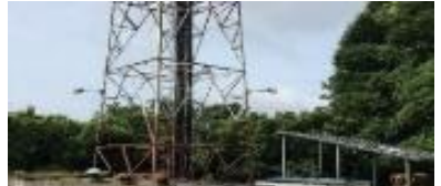
Energy-saving of mobile communications base transceiver stations, KDDI Corp. Indonesia
