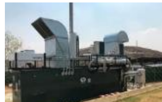
Power Generation with Methane Gas Recovery System, NTTDATA, Mexico
